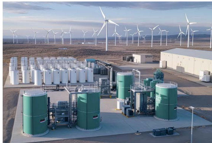
Large battery energy storage systems present new logistical, regulatory and safety challenges for heavy-haul transport operators.
